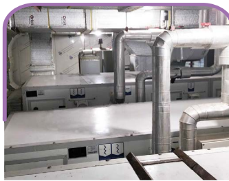
Air Handling Unit (AHU) for Environmental Control
