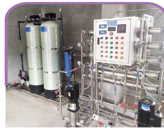
Highly efficient Water Treatment Plant with RO Process
